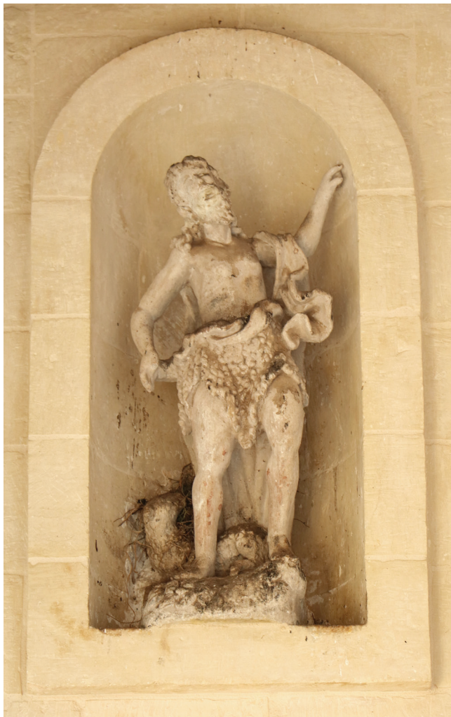
Fig. 4 Stone statue of St John the Baptist on the external façade, before restoration. (Photo: Restoration and Preservation Department, Malta)
